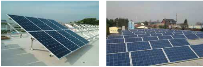
Figure 46: Typical flat roof installations
