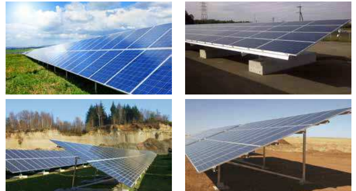
Figure 48: Typical on-ground field installations
