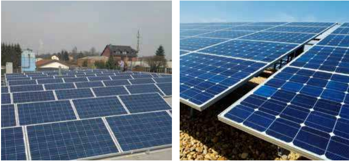
Figure 35: Installed PV modules
