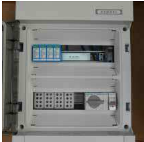
Figure 56: AC disconnection box including lightning and surge arresters, circuit breakers and main switch
