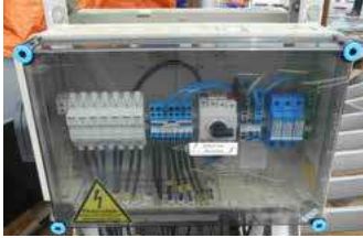
Figure 55: String combiner box in a solar power system
