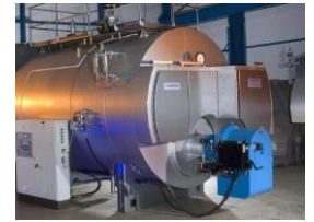
Preheating of Boiler Feeding Water
